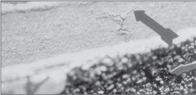
Photo 7. Close-up on bottom side of Tab A-5 of half-panel designation CO-WFB-D-7 at impact site. Note multi-line fractures radiating from common point.
