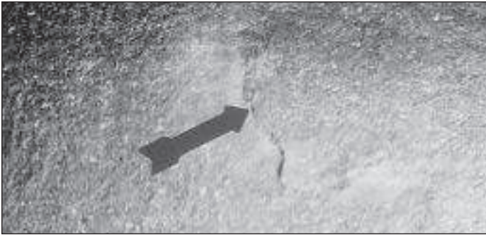
Photo 6. Close-up on bottom side of Tab D-4 of half-panel designation CO-FS-D-7 at impact site. Note curved-line fracture pattern weathered 4 years 4 months.
