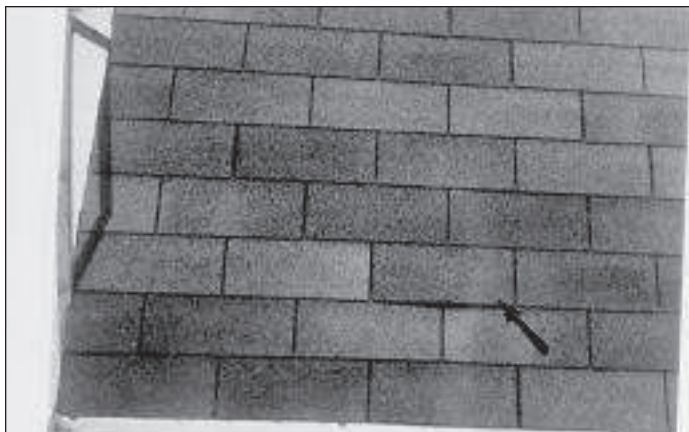
Photo A1. View of test panel at Year 0 before impacting. Note Tab G-3 at arrow.
