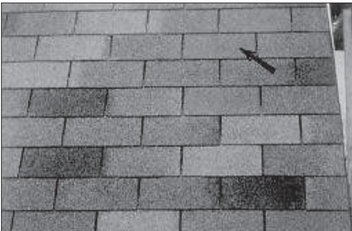
Photo C1. View of test panel at Year 0. Note Tab C-5 at arrow.
