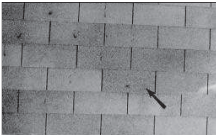
Photo A2. View of test panel at Year 0 after impacting. Note fracture in Tab G-3.
