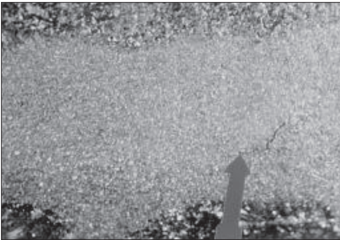
Photo D6. Close-up on bottom side of D-10 at location depicted in Photo D5. Note fracture.
